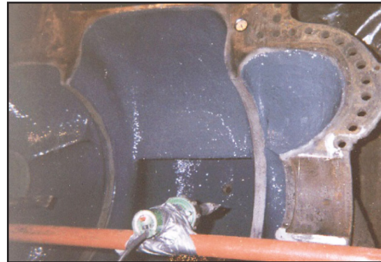
Split case fan pump, coated with ARC 855, ARC 858 and ARC 890
